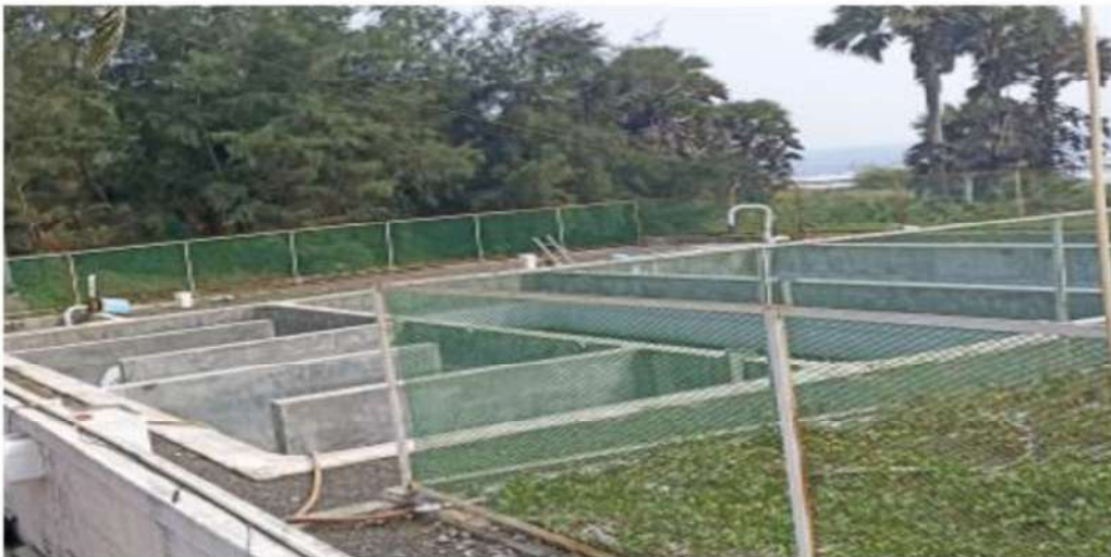
SEWAGE DISPOSAL TANKS
