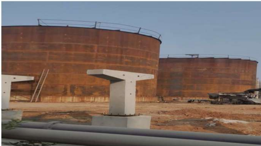
Sulphuric acid Tanks
